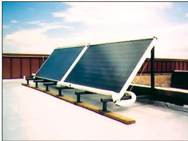
Figure 10: Solar Water Heating System.
